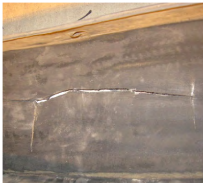
Cracked expansion gasket
